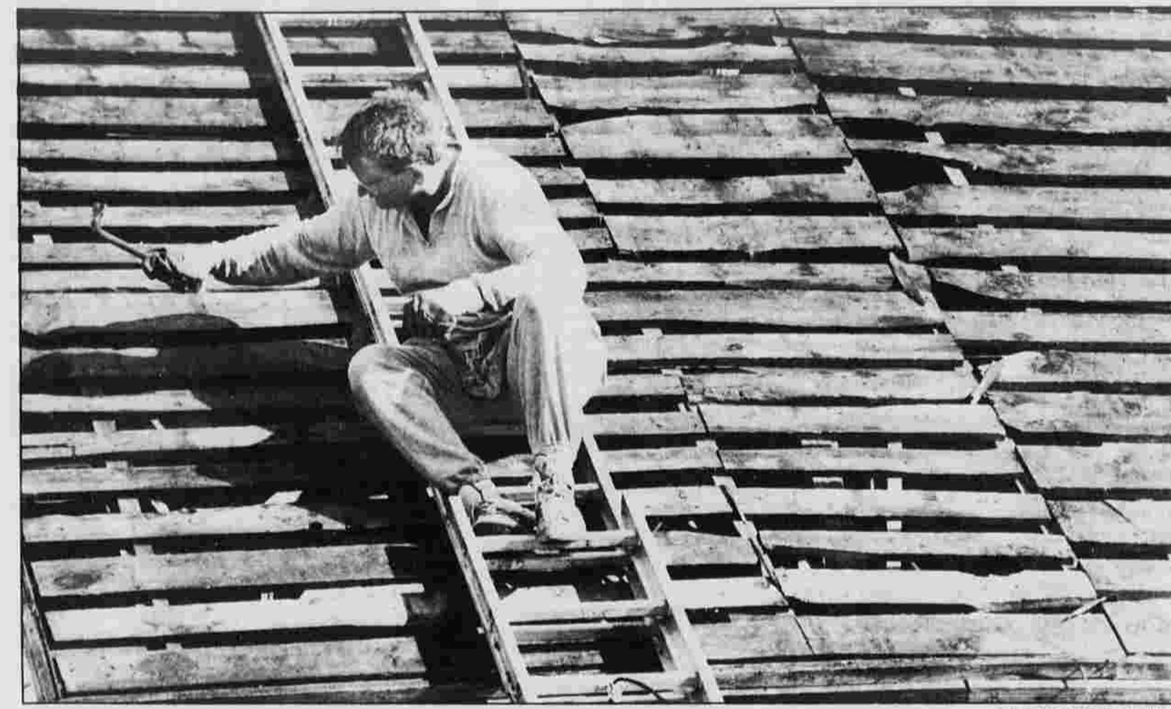
WEEKEND WORK — Kevin Murphy of 21 Stone St. sits atop his garage Saturday while performing a weekend repair project. He's installing a new roof. The National Weather Service says the weekend's sunny but cool weather will continue at least through Wednesday. That's good weather for outdoor work, like roof repairs and raking leaves.
